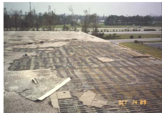
Figure 1. Roof cover failure Thomas Smith – TlSmith Consulting, Inc.
