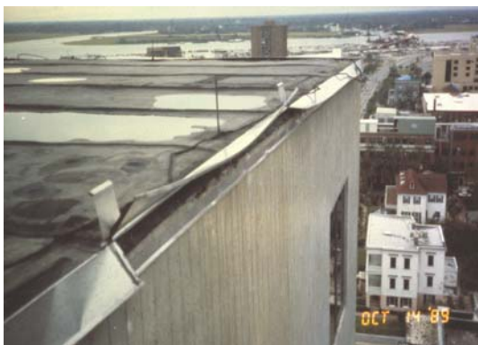
Figure 2. Perimeter roof flashing failure Thomas Smith – TlSmith Consulting, Inc.
