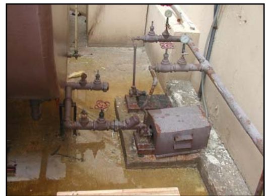
Figure 6. Fuel oil pumps within dike area of outside main fuel tank
