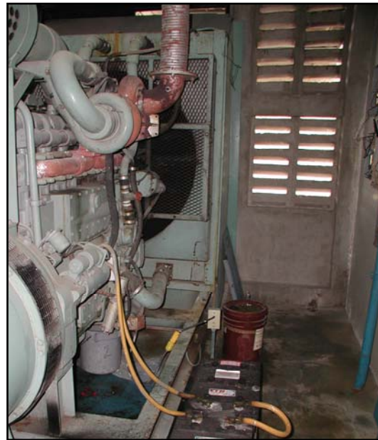
Figure 3. Combustion air louvers that allow carry-over of wind-driven rain
