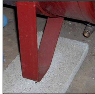
Figure 5. Fuel tank leg not bolted to floor
