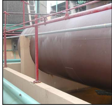
Figure 4. Outside main fuel tank secured against buoyancy by wrap-around concrete saddle
