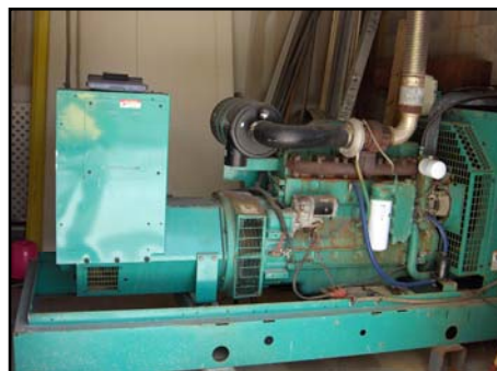
Figure 1. Diesel engine driven emergency generator
