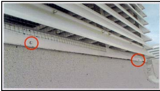
Inadequate securement Source – FEMA
