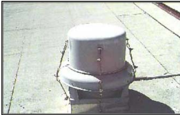
Secured fan and cowling Source - FEMA
