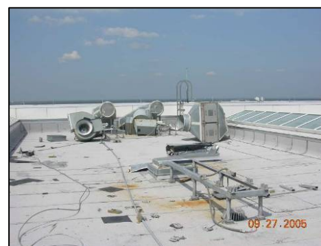
Wind damage to rooftop equipment Source – FEMA
