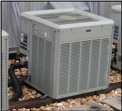
Limited attachment to unsecured wood blocking
