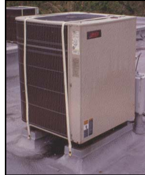
Well secured with straps, 2 screws desirable per strap connection Source – FEMA
