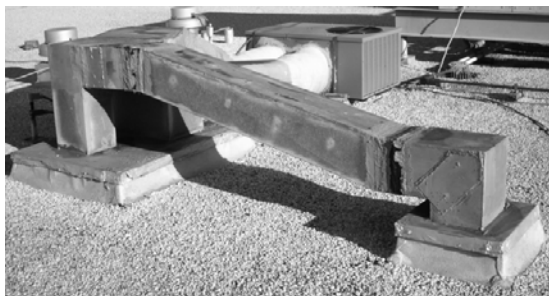
Exposed rooftop ductwork
