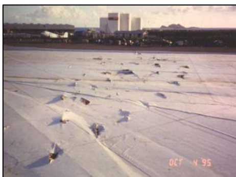
Roof cover damage from equipment Source – FEMA
