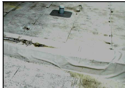
Ductwork installed under roof cover
