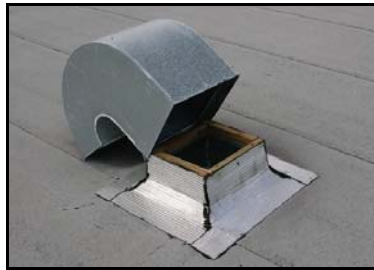
This goose-neck was secured with two screws. Failure lead to significant water entry into the building Source - FEMA
