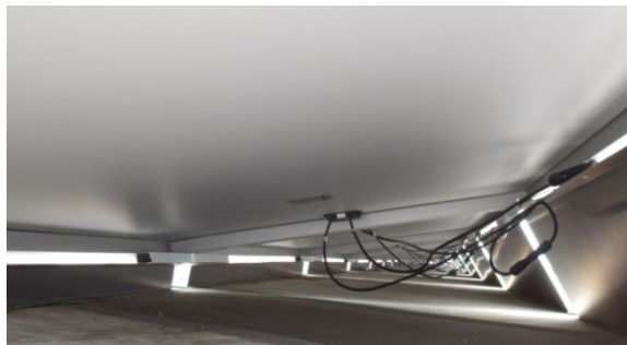
Figure 6 - Shielded area below photovoltaic modules (Photo source: Rich Gallagher, Zurich)
