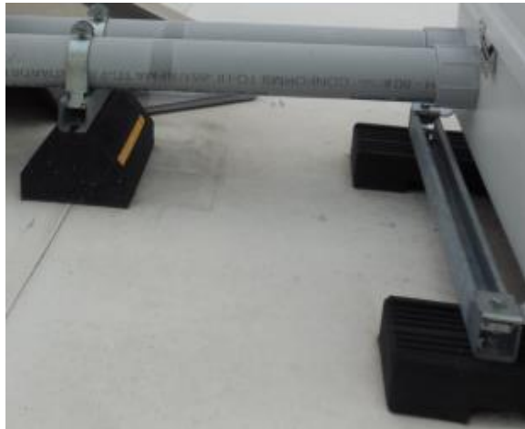
Figure 5 - PVC conduit and rubber support blocks (Photo source: Rich Gallagher, Zurich)
