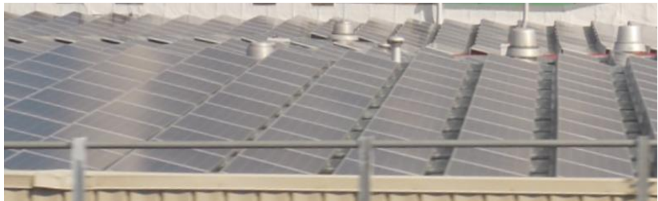
Figure 1 - With the installation of photovoltaic modules, in this example, the presence of rooftop electrics expands considerably compared to the pre-existing rooftop fans (Photo source: Rich Gallagher, Zurich)
